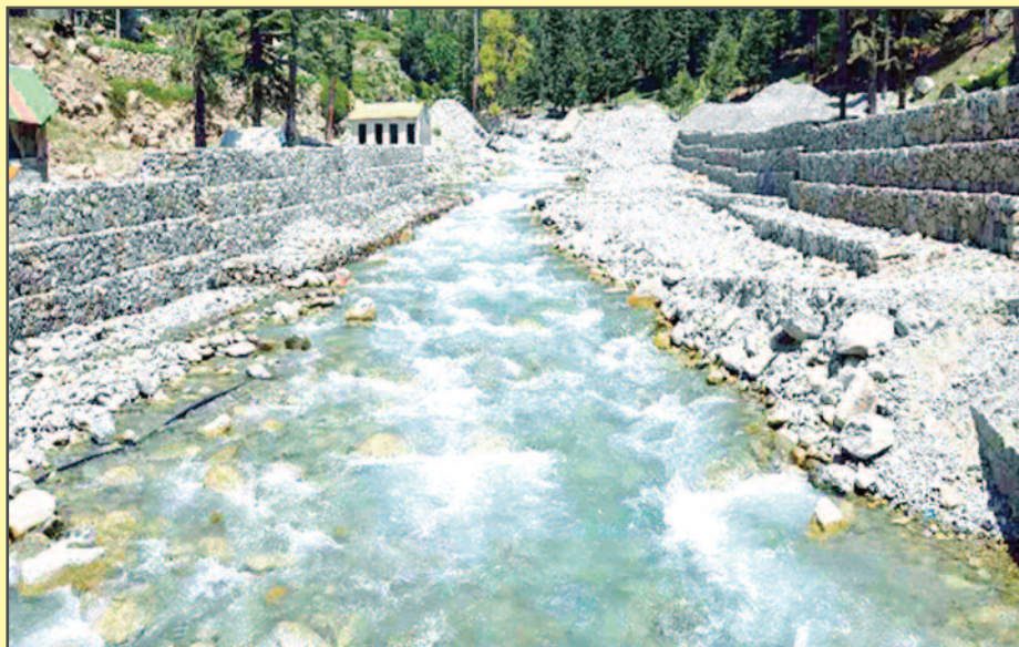
A view of the gabion wall constructed on both sides of the river by GLOF-II project of UNDP to protect the local population and hotels in Paloga area of the scenic Kalam valley.
