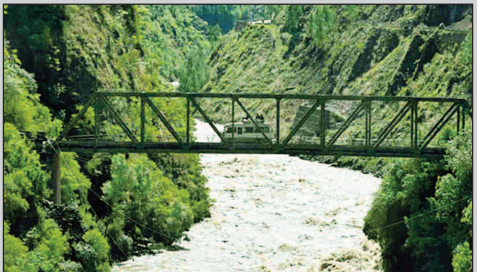
A bus crosses the half-a-century-old Neeli Bridge, one of the only access points to the Leepa Valley in Azad Kashmir.
