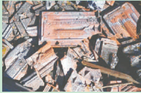
This photograph shows dozens of roof tiles lying on the floor, next to the frame of an ancient building of Antakya, with characters written on their back suggesting they were used during the French mandate over the city.
